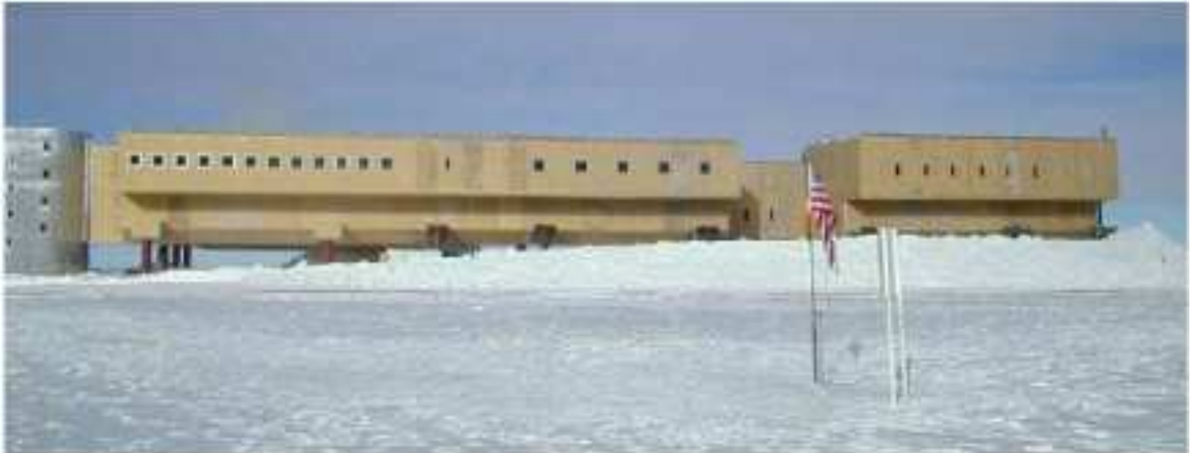
Figure 26: Construction of the new South Pole Station as of February, 2002. [From http://www.amanda.uci.edu/. ]
